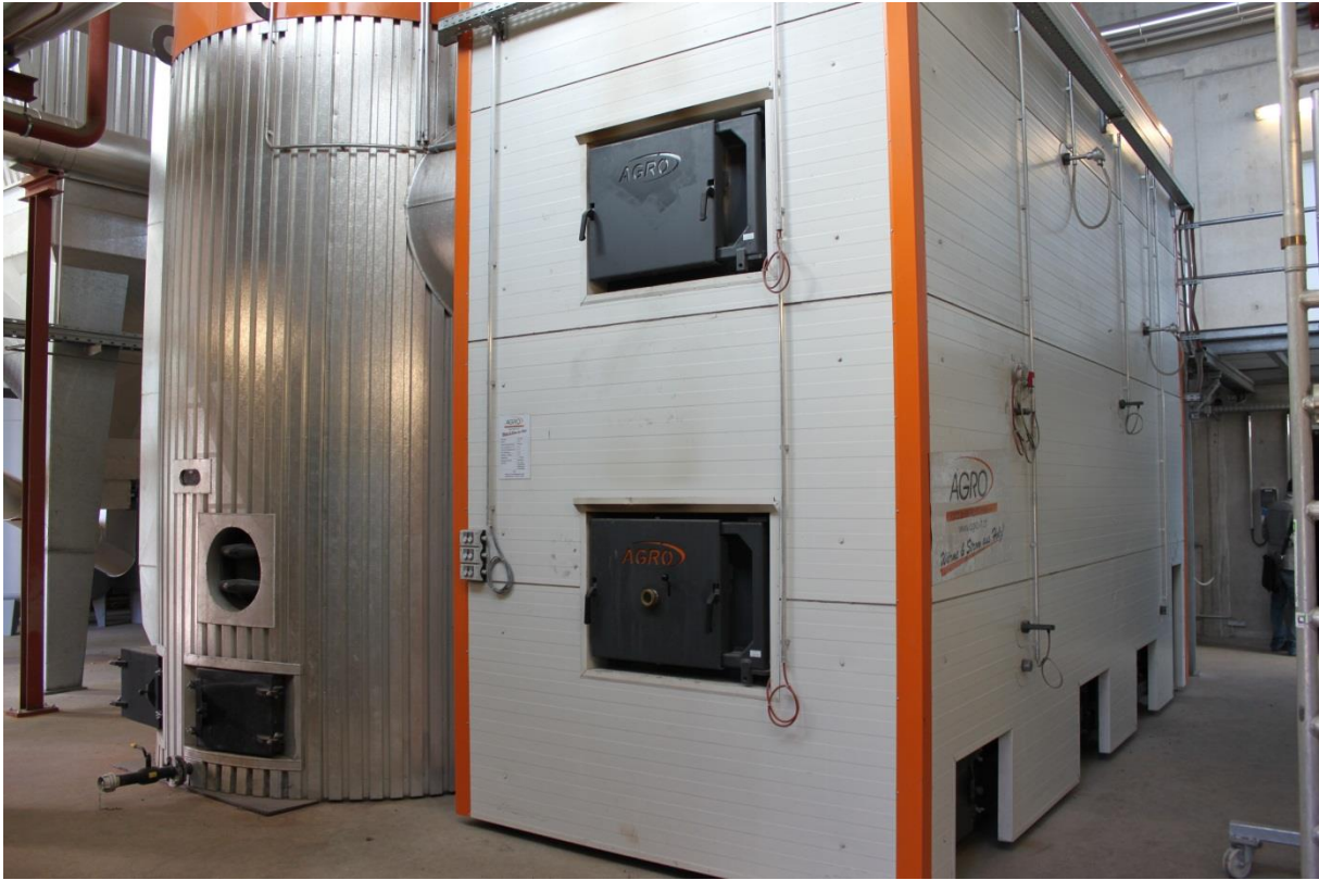
Figure 62: Medium sized woodchip heating system (3,000 kW heat capacity) with the boiler (right) and the buffer tank (left) of the Biomassehof Achental in Germany (Source: Rutz D.)
