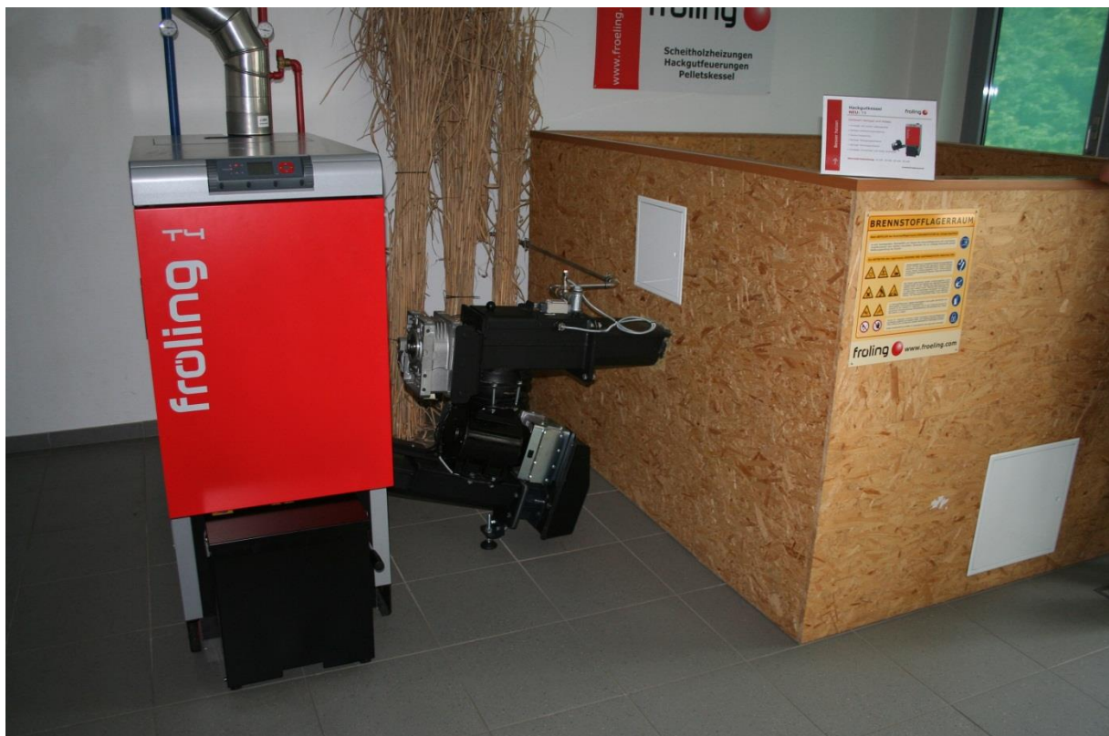
Figure 61: Small woodchip heating system (24-50 kW heat capacity) with the boiler (left), the feeding system (middle) and the woodchip storage (right) of Fröling (Source: Rutz D.)
