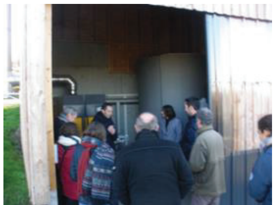
Photo 2 : The group visiting the boiler and the hot water tank.
