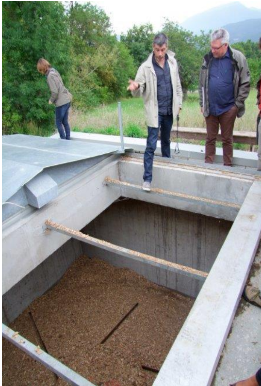
Picture 6: Visiting a wood chip heating system (heating municipal buildings, the library and 3 council flats) in Le Percy
